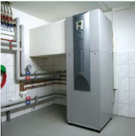
Air/Water Compact heat pump indoor installation 6 kW
