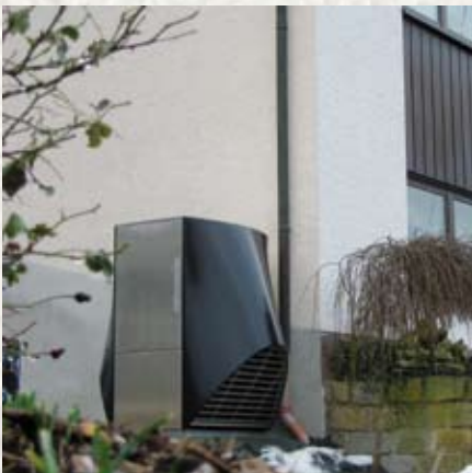
Air/Water heatpump outdoor installation 33 kW
